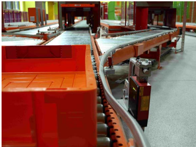
Figure 2. Route choices in the extensively branched conveyor system are made by reading barcodes.
