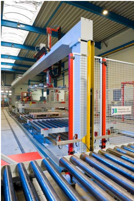
Figure 2. CPSET in a handling system for the wood industry
