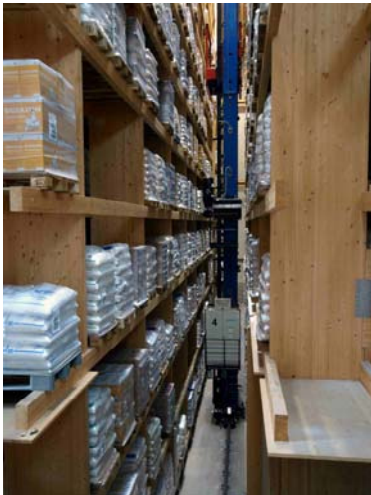
Figure 1. Wood is an unusual building material for a high-bay warehouse. For the Salinen Austria AG salt warehouse, however, it is ideal.
