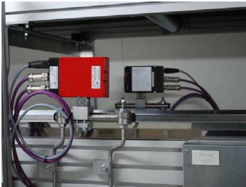
Figure 6. Barcode readers on the transport path read the preset codes as the containers pass through and transfer the data to the control via PROFIBUS.
