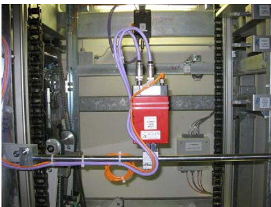
Figure 5. The inner workings of the vertical conveyor contains highly dynamic drive elements and reliable sensors at the PROFIBUS.
