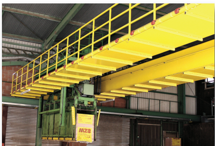
Diffuse reflection light scanners on the gantry crane monitor the transfer station from above to locate unoccupied storage spaces.
