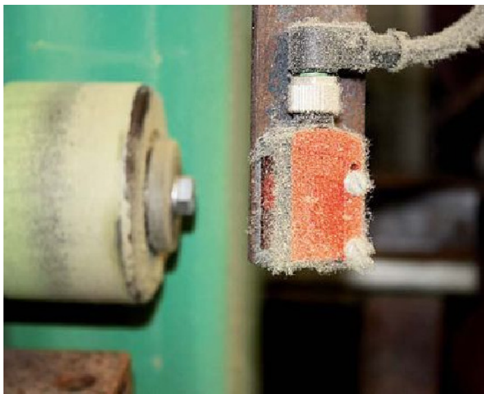
ABOVE: The dust that is created when cutting the rock wool mats for the ThermoPlan MZ8 does not affect sensor function
